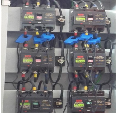
Figure 4: Six CTs connected at 3-phase air conditioner load
